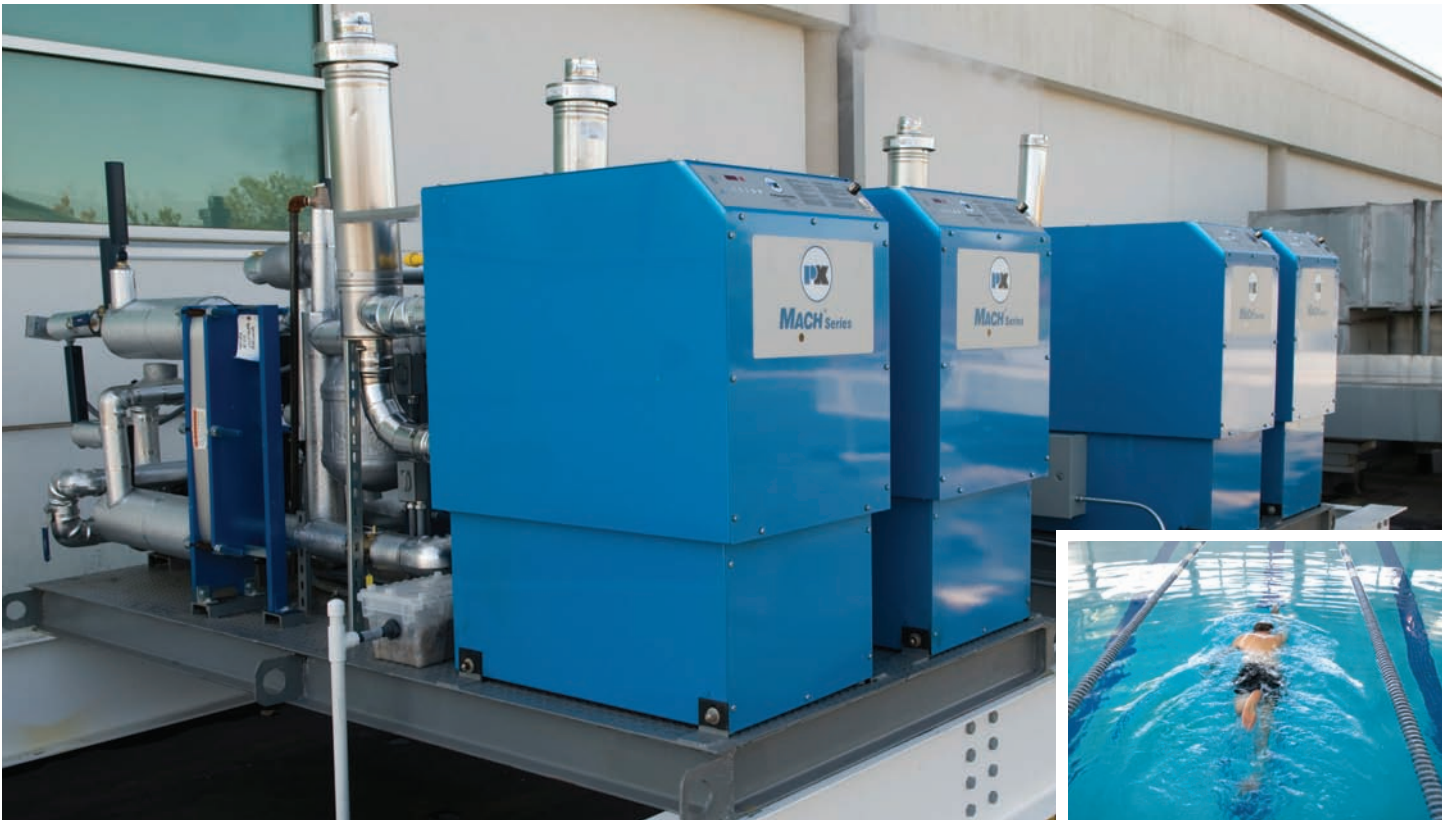
Pictured above is an outdoor installation of high-efficiency condensing natural gas hot water boilers manufactured by Patterson-Kelly.
